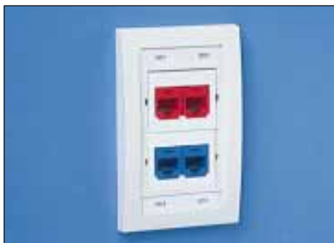
Network Systems Labeling
