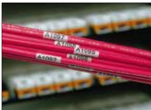
Wire and Cable Identification
