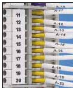
Terminal Block Labeling
