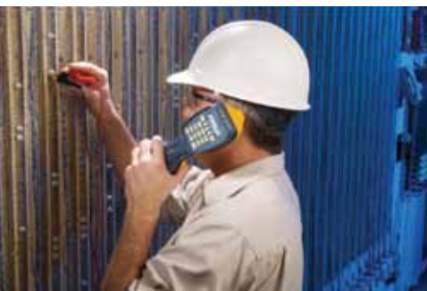
Telephone/Data Room or Central Office
