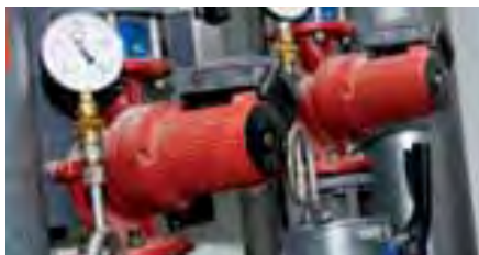
Actuators, valves, control cabinets
