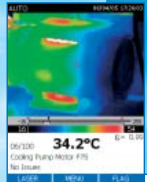
Cooling pump running at operating temperature.
