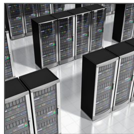
Data Center Servers
