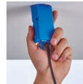
Simple spotlight installation
