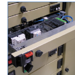
Equipment with TeSys T motor starter
