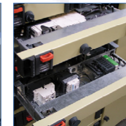
Equipment with TeSys T and TeSys U motor starters
